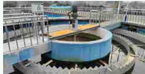
Yangcun Coal Mine domestic sewage treatment system
