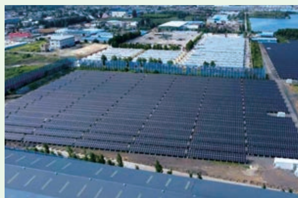
Distributed photovoltaic panel in Xinglongzhuang Coal Mine
