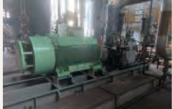
New turbine generator sets to the methanol synthesis device
